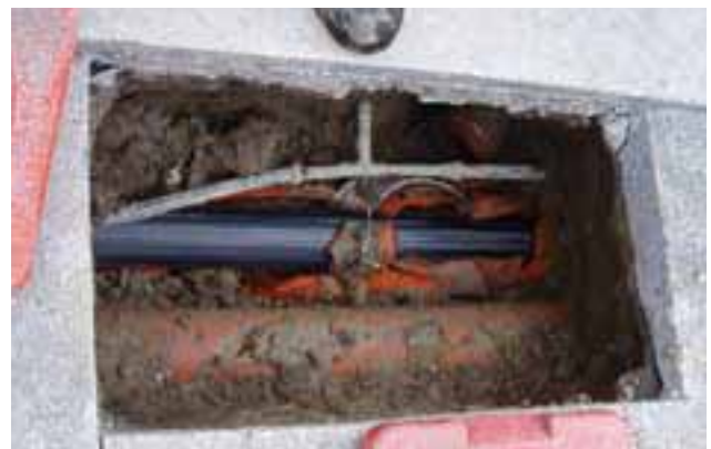
Above: A new plastic pipe being inserted through an existing private sewer drain.
