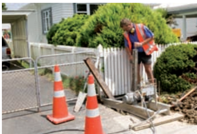
Above: Alan Perkinson of Perkinson Civil connects a new pipe to the mains as part of the upgrade work carried out in Area 1 during February.
