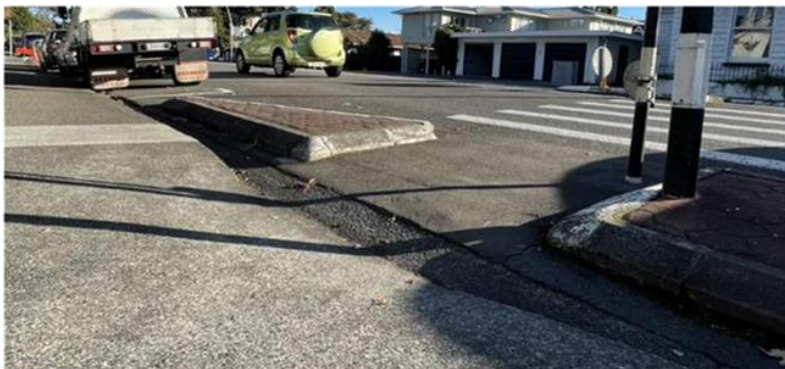
Figure 3: Steep footpath ramp and no tactile pavers at Bloomfield Terrace
