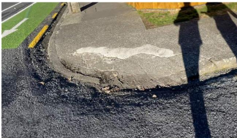
Figure 2: Poor footpath ramp surface at Willoughby Street with no tactile pavers
