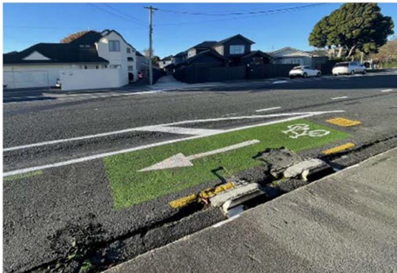
Figure 2-13 Damaged pavement outside 142 Knights Road
