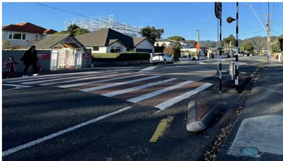
Figure 7: Poor conspicuity of the zebra crossing
