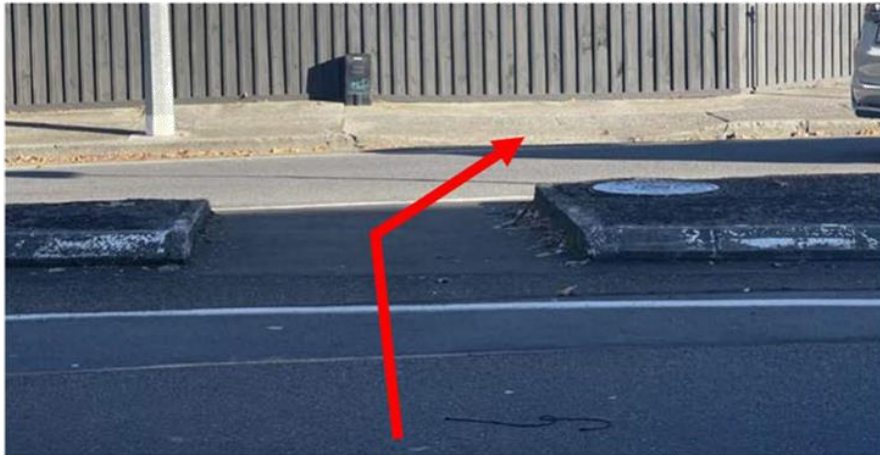
Figure 11: Misaligned pedestrian crossing on the eastern Knights Road approach
