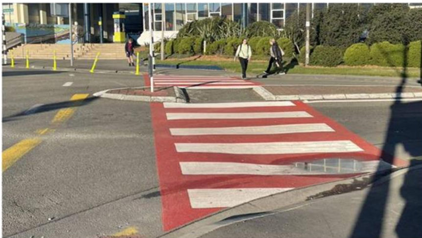
Figure 14: Slumping pavement surface leading to ponding at the Pohutukawa Street intersection
