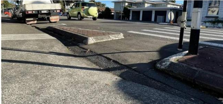
Figure 9: Steep pedestrian ramp and pavement lip at the southern pedestrian crossing
